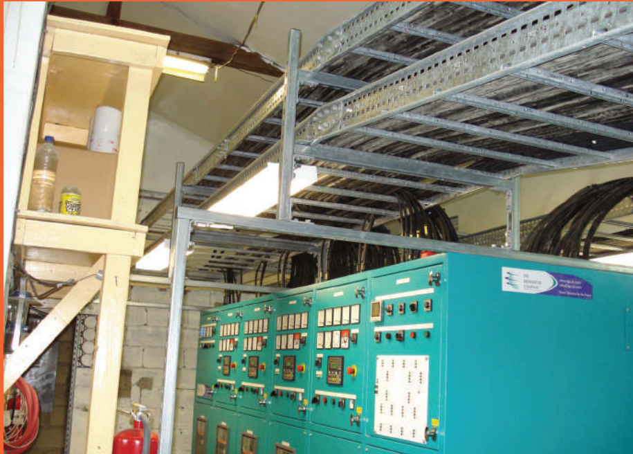
Switch Room after modification
