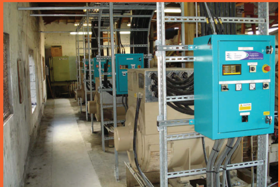
Generator Room after modification
