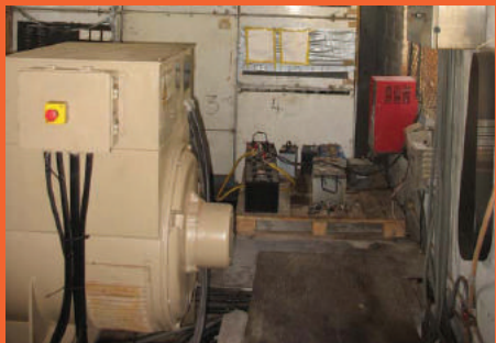
Original Control System Installation
