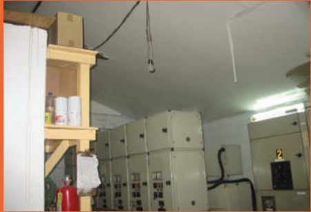
Original Yorkshire'YSF6 MV Switchboard
